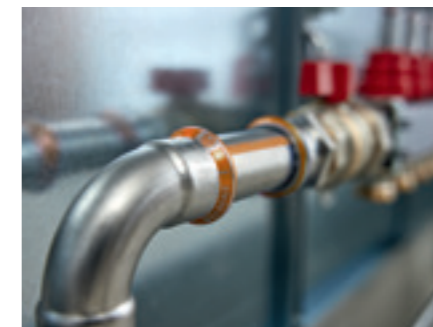
Additional marking with the 'non-potable water' warning sign
